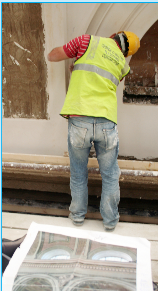
One of the professional plastering team at work at trial plasterwork in July.
